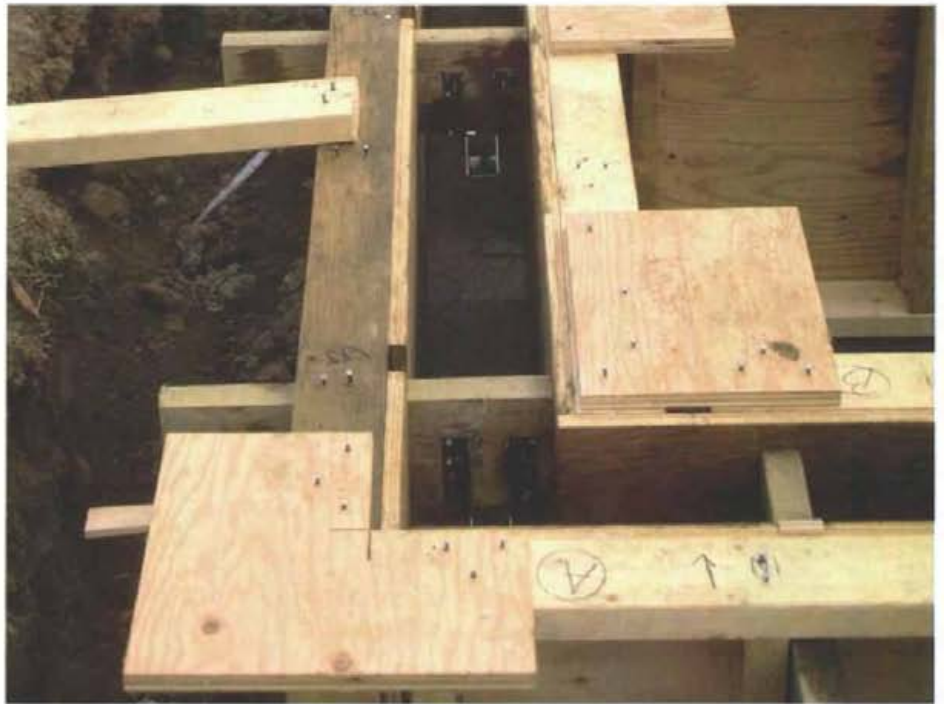
Thinking ahead. Lookouts embedded in the concrete (and held securely by the addition of a joist hanger nailed to each side) provide rock-solid support for the first tread of the step that runs around the porch's perimeter.
