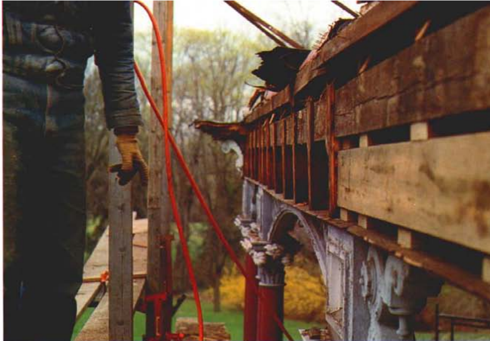
To make the lintels look beefier than they are, the original builders dropped the lintel soffit nearly a foot below the lintel and framed in the space between the lintel and the soffit with 2x6 cripple studs. The author replaced the studs beneath each damaged section of the lintel with a 6x8 beam (at right in photo), adding blocks to transfer the load.
