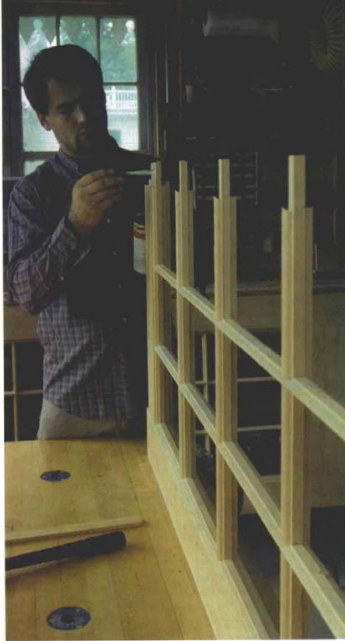
A paintbrush spreads an even coat of glue. After dry-fitting, an exterior-rated wood glue was applied to the mating surfaces of the door, which were then clamped.
