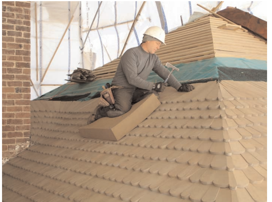
Old-growth cypress shingles were laid over new spaced battens to restore Montpelier's roof surface. The green membrane is Roof Shield, and the black mesh just above the shingles is Cedar Breather. A swept valley is visible behind the chimney at left, and a fanned hip appears on the right. The carpenter's foam rubber cushion protects shingles during installation.
