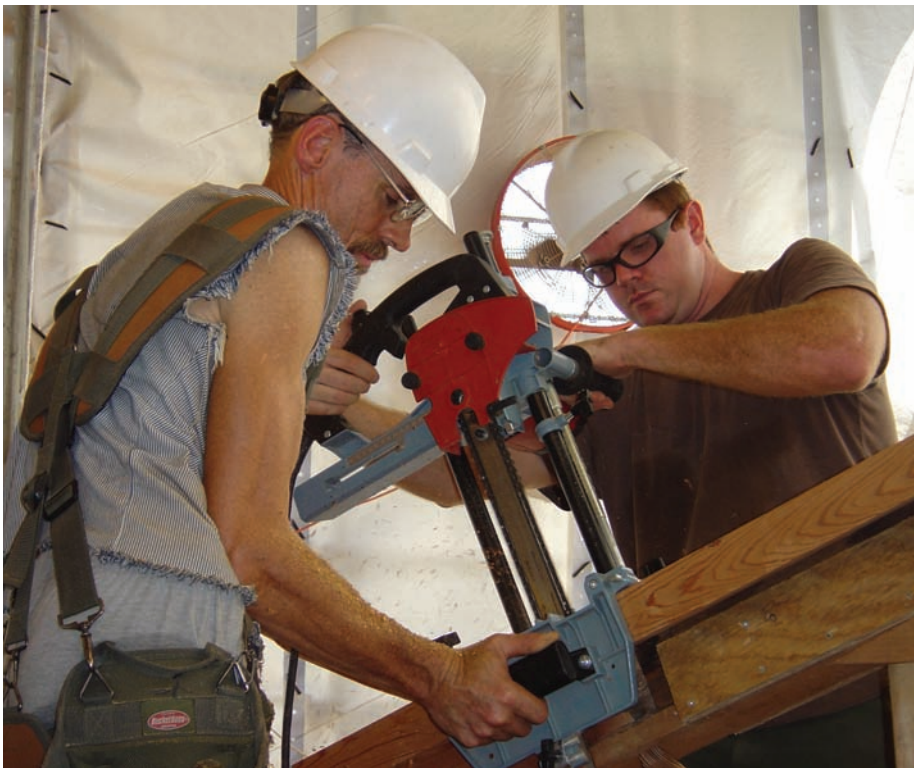
A spliced hip rafter was grooved with a chain mortiser to receive internal steel knife plates. Photo: Amy Wysocki
