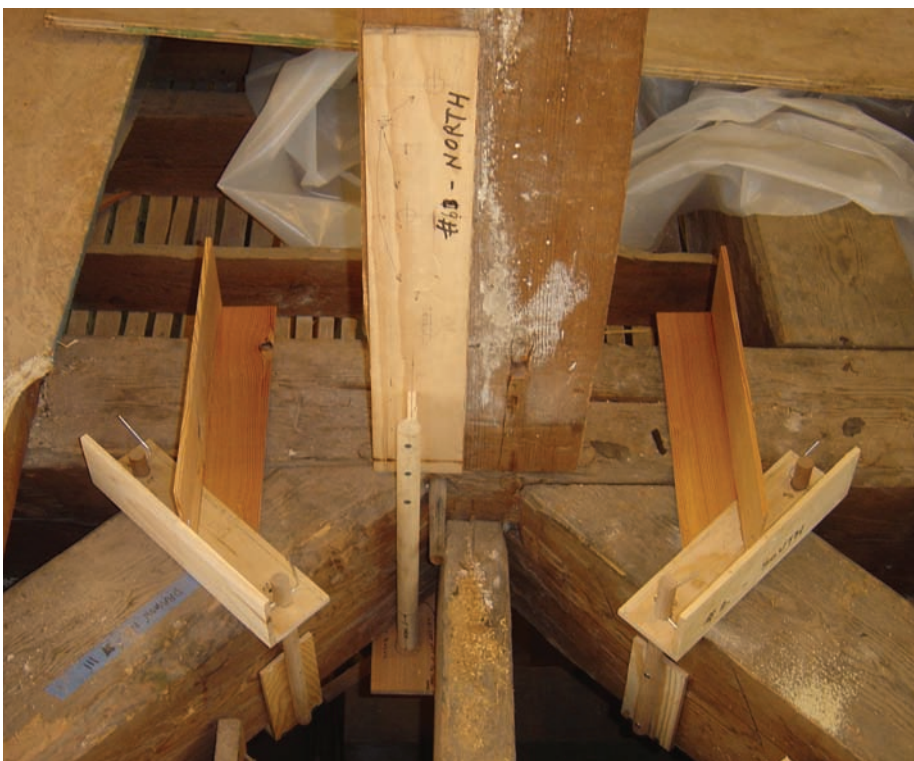
Two dragon beams, a joist and a kingpost all converge at the midpoint of the principal roof truss. The resulting mortises weakened the lower chord of the truss to the point of failure. After jacking up the truss, wooden patterns were made for specially designed steel hangers. Photo: Amy Wysocki
