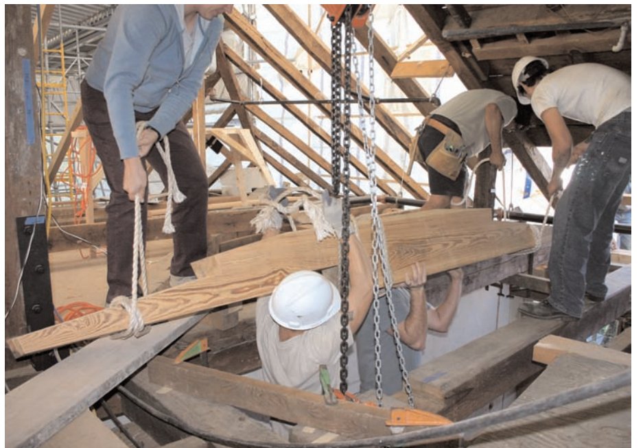
One of the beams that ties Montpelier's portico to the house had rotted clean through, so a 12-ft. section in the middle had to be replaced. Bolted scarf joints united replacement material with the original fabric. Reclaimed heart-pine timbers were salvaged from a textile mill in South Carolina. Photo: Maggie Wilson
