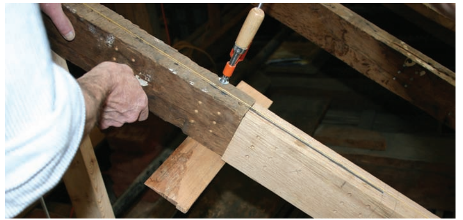
This 18th-century rafter (left) was severed in 1901 to accommodate roof alterations. A new extension (right) was attached by means of an internal steel knife plate that bridges the joint. The plate drops in from the top and is secured by four sets of self-drilling steel pins. Photo: Maggie Wilson
